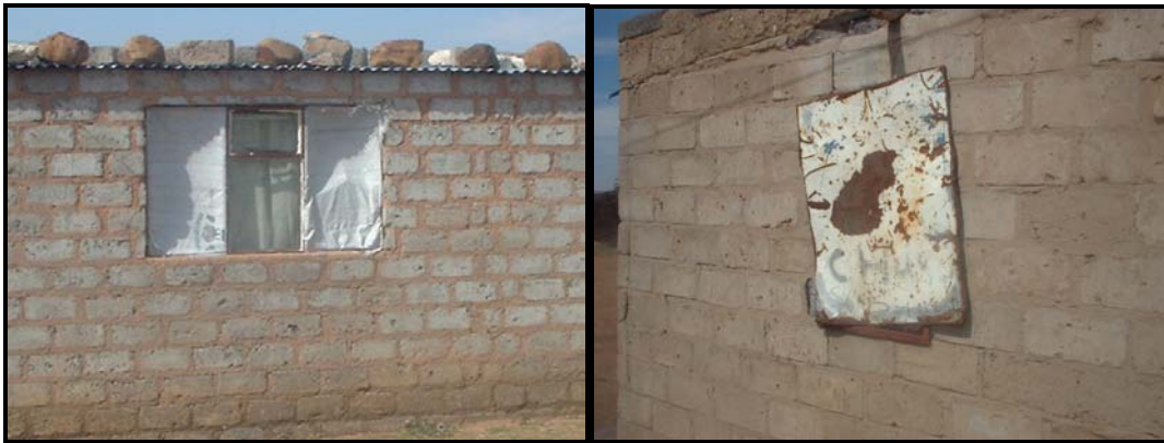
Figure 5 Non functioning windows that have been covered
